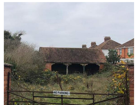
Existing dilapidated single storey building within the site.
